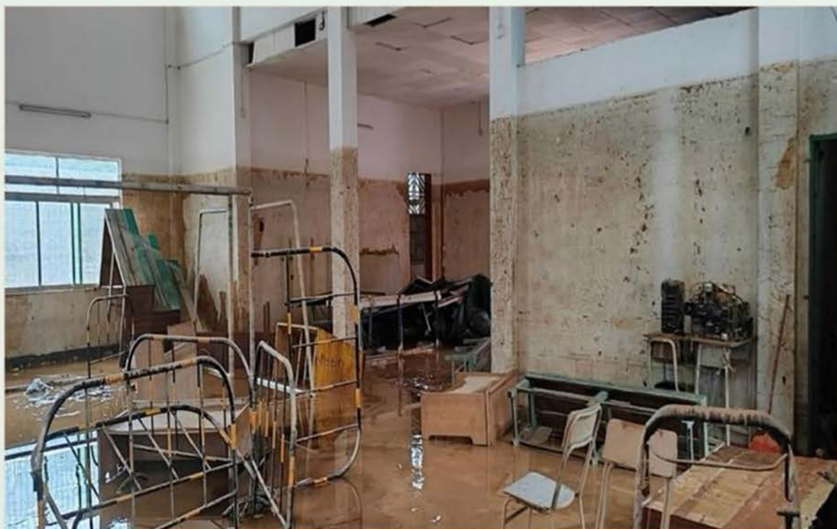
Baidu Middle School was submerged under 3 meters of floodwater, resulting in severe damage to its facilities.
